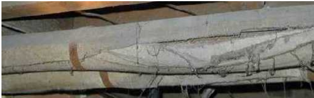
The above photo shows a typical asbestos insulated heating pipe found in older homes.
